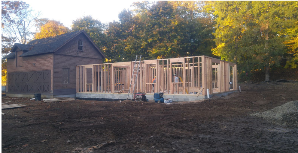
New Grover Cleveland Birthplace Visitor's Center, November 6th, Framing of exterior walls complete. (Courtesy of Sharon Farrell, Grover Cleveland Birthplace Caretaker, State of New Jersey.)
